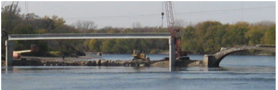
New Evansdale Bridge on left replacing the old bridge on right - October 2010
